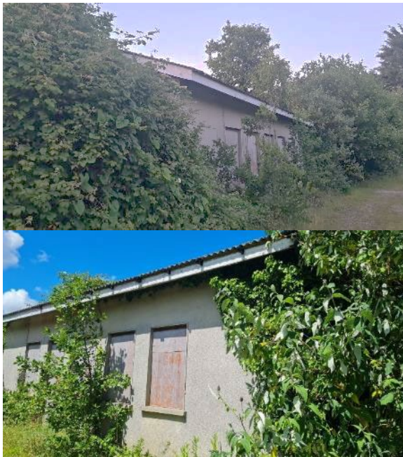
Building 8, overgrown shed
