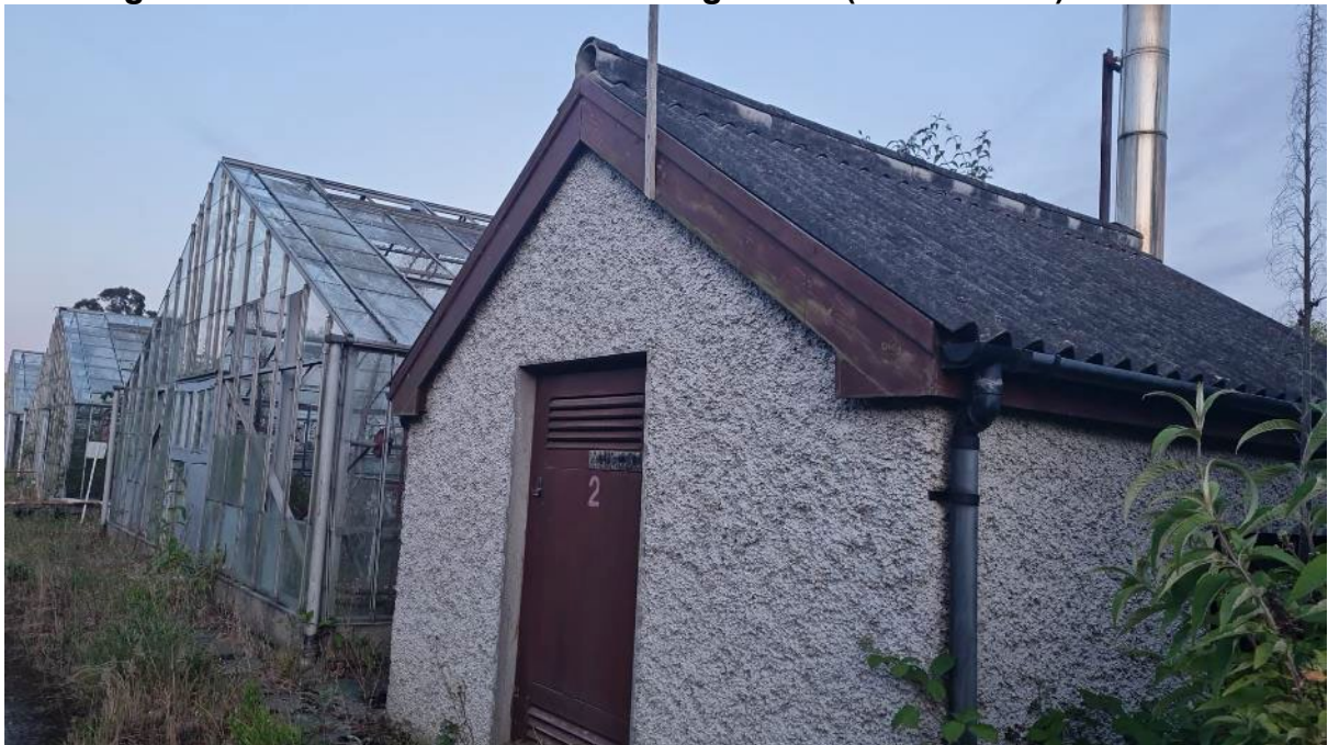
Building 10 Water supply at greenhouses
